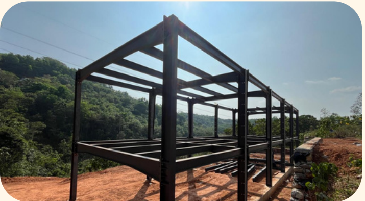
As of March 2026, the fabrication of the steel structure for the administration block has been completed.
